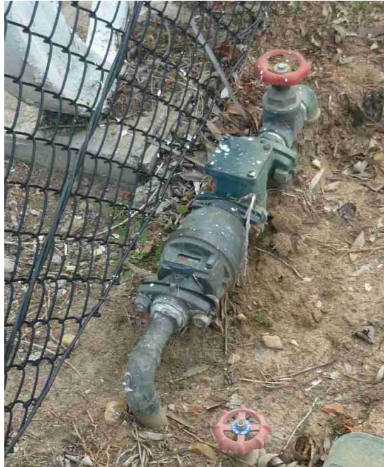
Figure 1. The Main Water Meter at Wodonga Caravan and Cabin Park
